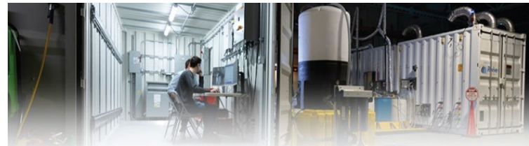
Destroying Forever Chemicals with PFAS Annihilator™
